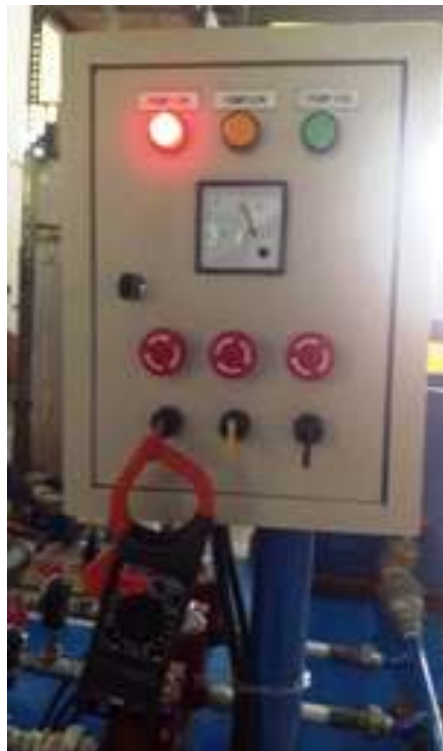
Gambar 3.3. Panel kontrol pompa
