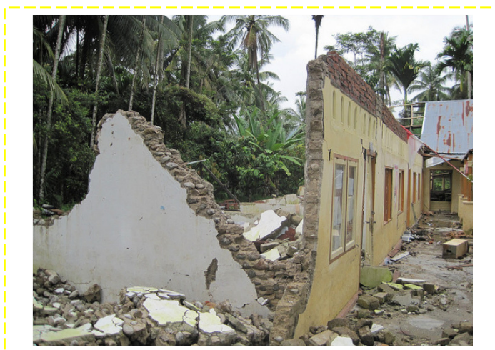
Figure 6. Buildings in Padang, Indonesia after earthquake September 30, 2009 (7.6 on Richter scale). Damages to an unconfined single story school building.
